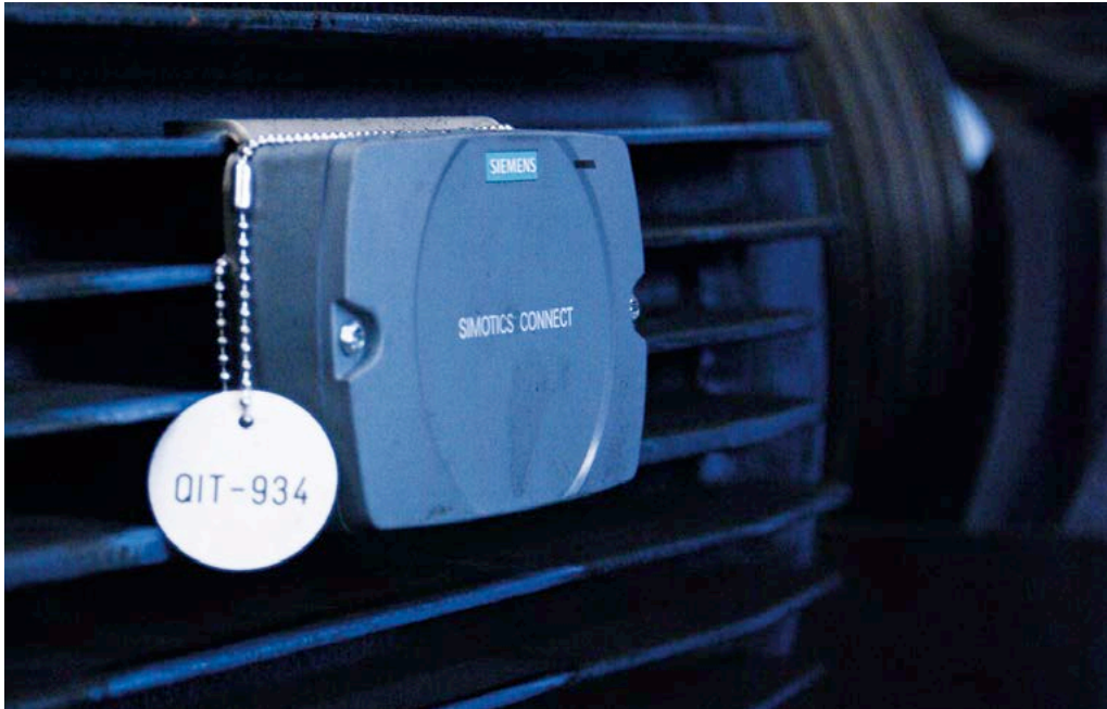
SIMOTICS CONNECT 400 (SC400) mounted on one of the aerators in a wastewater treatment plant of Scottish Water.
