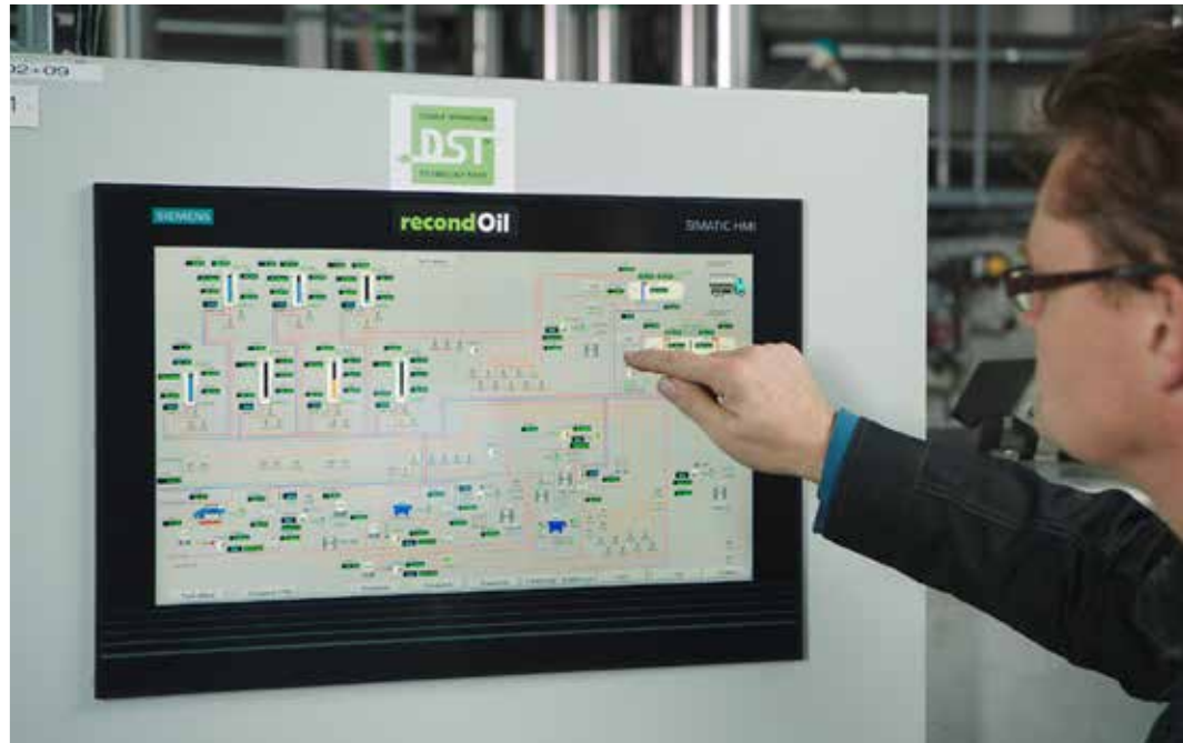
SIMATIC S7-1500 control system integrates the data collected by process instrumentation in a centralized location for operators to have easy access to their plant systems.
