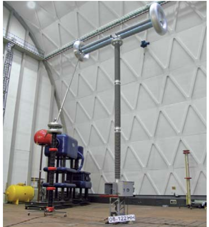
Figure 3: High voltage test of an 800 kV Pole
