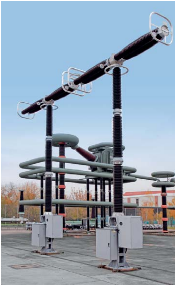
Figure 1: Breaker pole on the new 800 kV outdoor circuit-breaker
