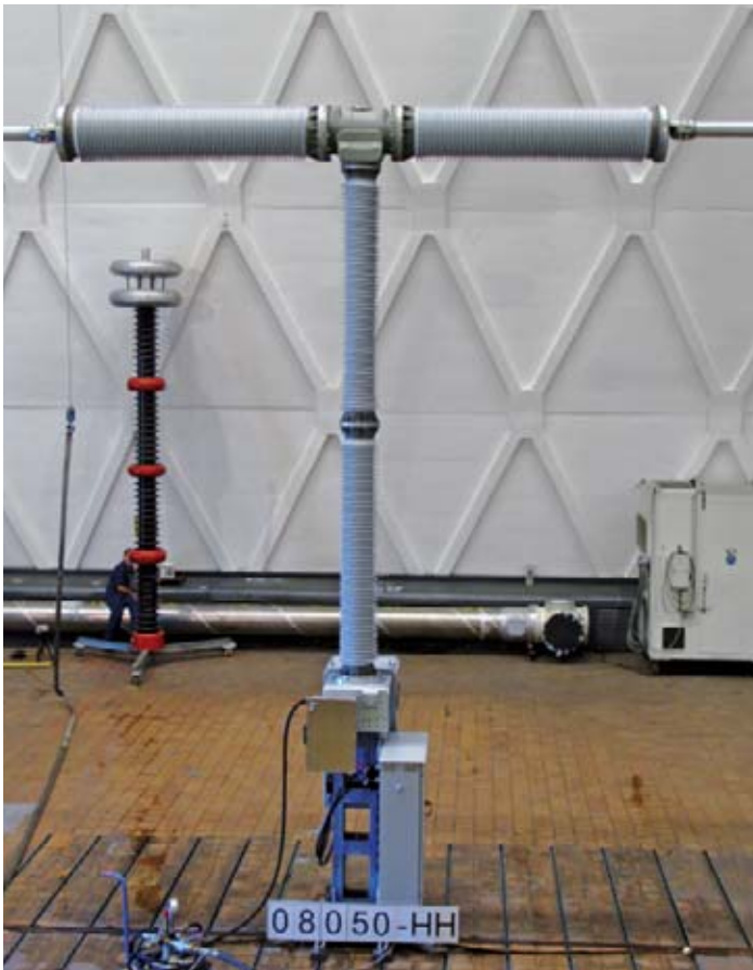
Figure 11: 420 kV disconnecting circuit breaker pole
