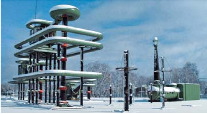
Figure 3: 1800 kV Transformer in the outdoor test station
