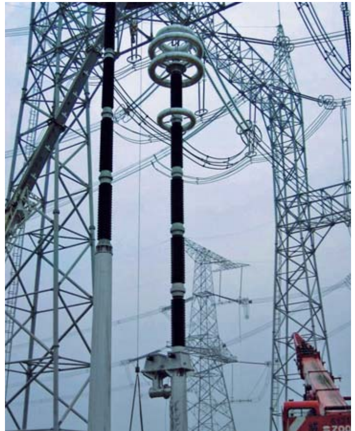
Figure 11: Capacitive voltage transformer in an 1100 test setup at Wuhan/China
