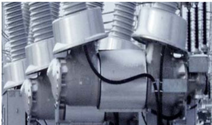
Figure 2: Use of a tank heater on a dead-tank circuit-breaker, type 3AP1DT - 245 kV
