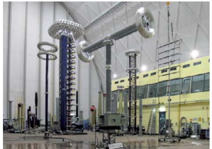
Figure 4: High voltage test of a 400 kV Pole
