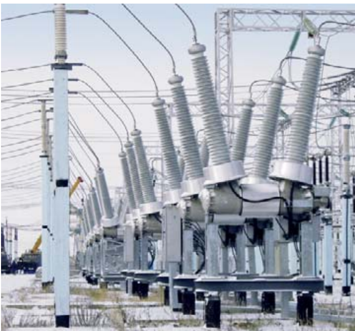
Figure 4: Installation and commissioning of a dead tank circuit-breaker for 245 kV in Sokol, Kazakhstan
