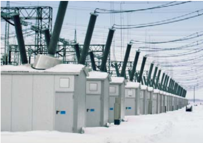
Figure 3: Installation and commissioning of a dead tank circuit-breaker for 550 kV with heatable thermo housing in Sokol, Kazakhstan
