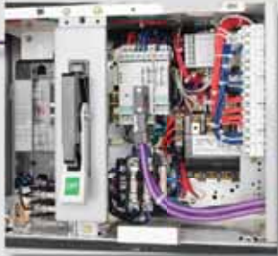
FVNR starter installed with SIMOCODE Pro V
