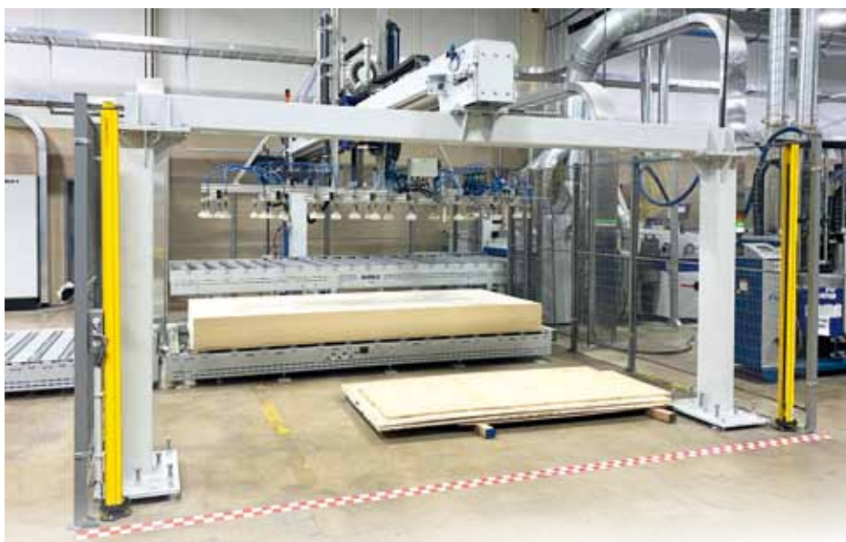
Installed gantry feeder with protection board storage. Positioned in front of a panel cleaning and coating system at a renowned panel finishing company. Version as seen in the CAD drawings (1 to 3)
