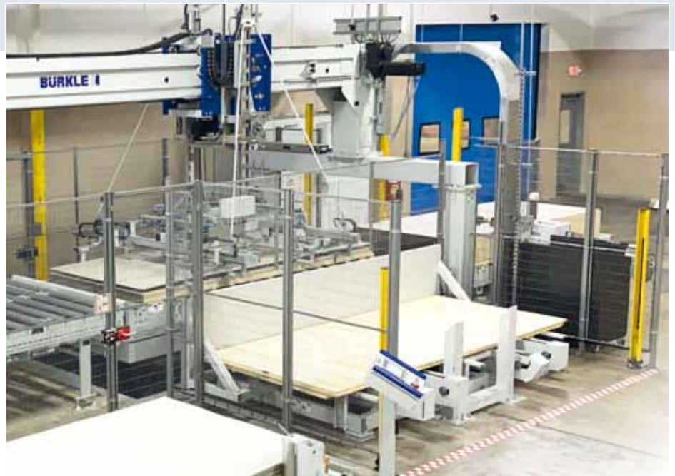
After installation and commissioning. Side view of panel de-stacking with protection board feed (middle) and exit position of the finished stacks (concealed at the rear) with panels passing through
