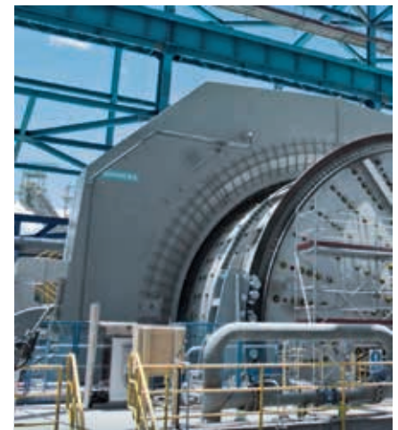
New greenfield processing plants are once again being built to process higher volumes of extracted ore.
