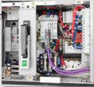
FVNR starter installed with SIMOCODE Pro V
