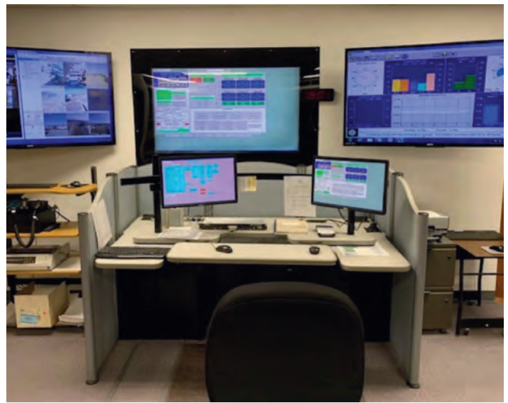
Control room with two operator stations.
