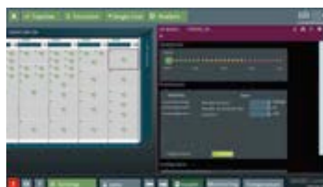
Low-voltage switchboard – Health status
