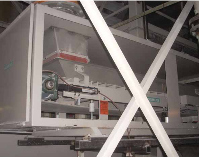
Installing and testing SITRANS WW200 was a simple process. NOPA's operators have been pleased with the weighfeeder's reduced maintenance requirements.
