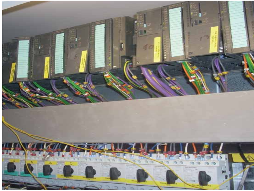
SIWAREX FTC weighing modules provide fast, continuous monitoring and control delivered directly to NOPA's control room.
