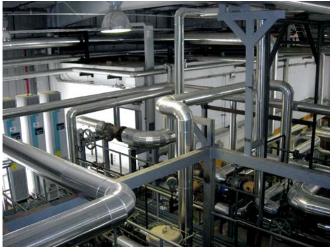
Fig. 1: Piping for SCHEITER® hot water plant with recovery system including all secondary plants for the tire industry
