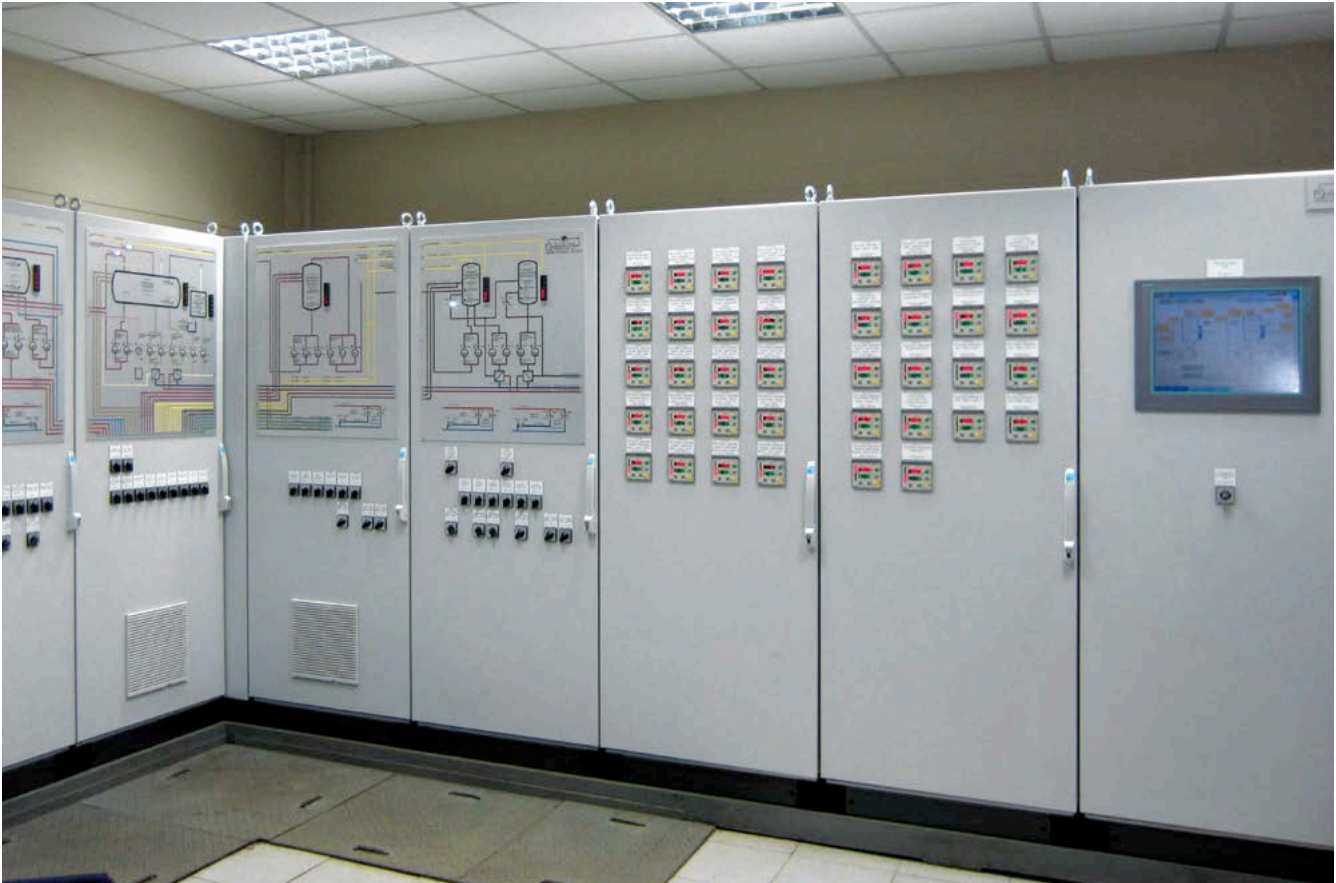
Fig. 3: Switch board for SCHEITER® hot water plant with recovery system including all secondary plants for the tire industry
