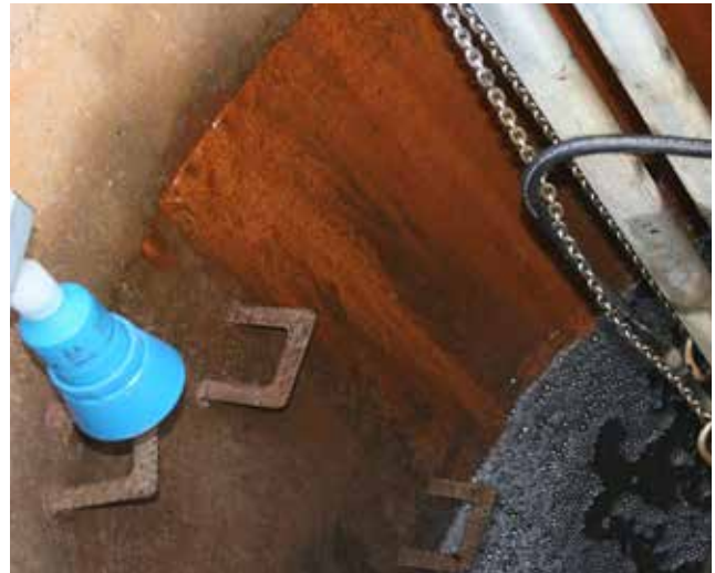
Siemens Echomax transducers installed in the well and the SITRANS LUT400 controller measure the level of water and control pump operations.
