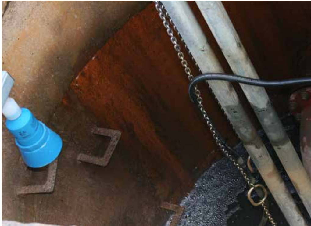
With the numerous obstructions in this wet well, including a ladder, pipes, and chains, accurate and reliable level measurement can be quite challenging.
