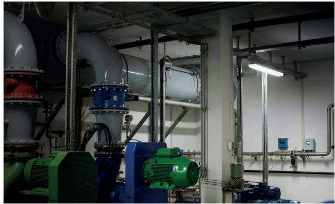
Safety under the most demanding conditions: From now on, the digital clamp-on ultrasonic flow meter ensures high-accuracy flow measurement of the return-activated sludge.
