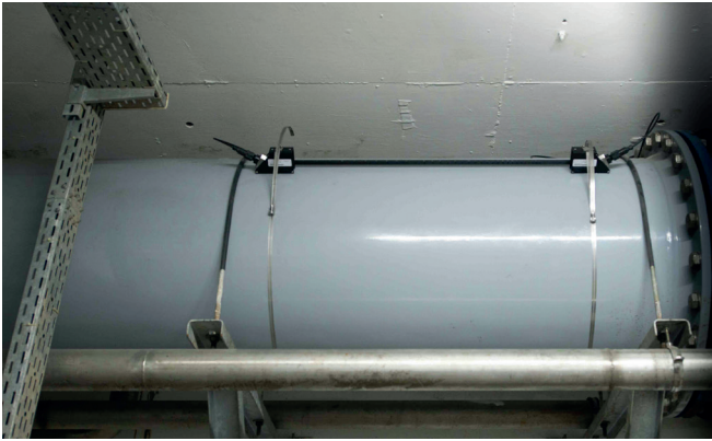
Siemens clamp-on sensors mounted on a 32 in steel pipe to measure the return-activated sludge.
