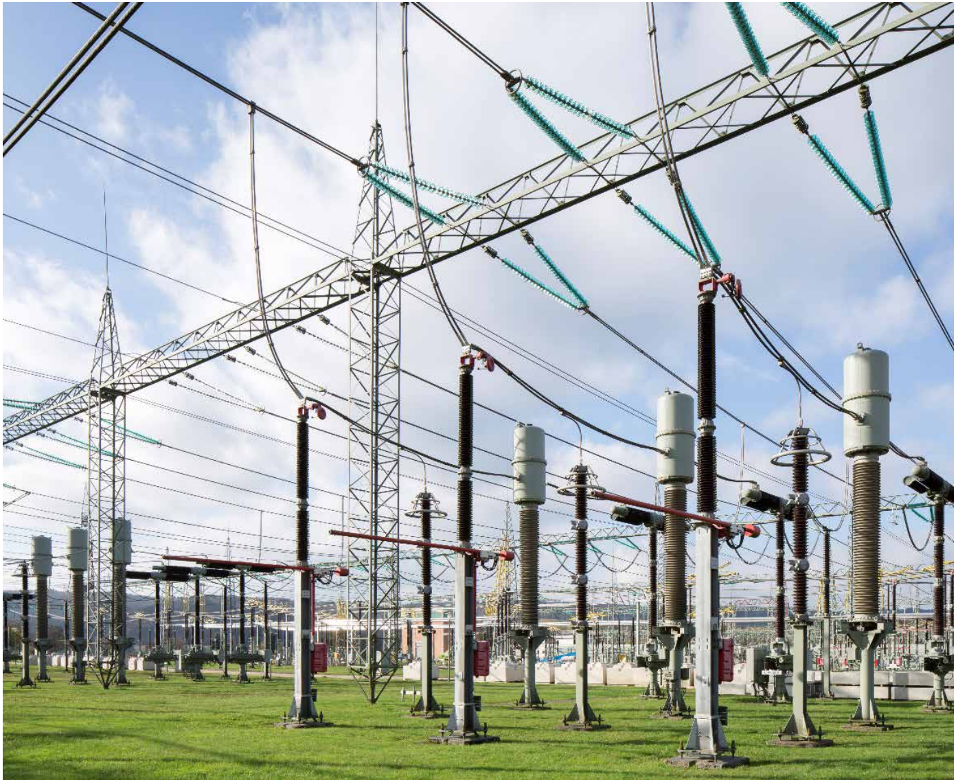
Planned based on a similar principle, Amprion's substations play a key role in transmitting power to approximately twenty-nine million people in Germany.
