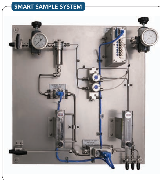
Figure 1. This sampling system includes sensors for pressure, temperature and flow.
