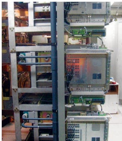
New interface boards for the SINAMICS drive control fixed at existing power stack tower
