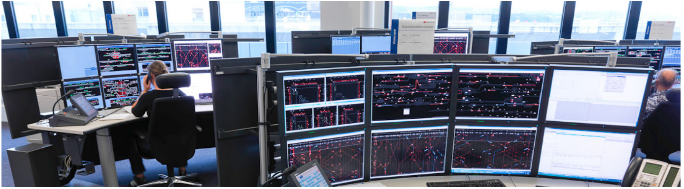
Controlguide® Iltis N operation centre
