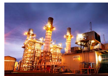
Main application: Industrial power generation
