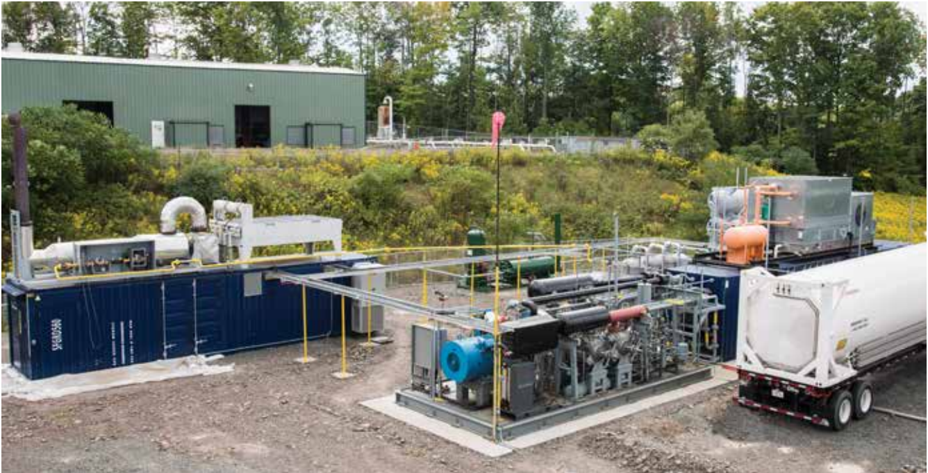
LNGo system installed at the Ten Man compressor facility.
