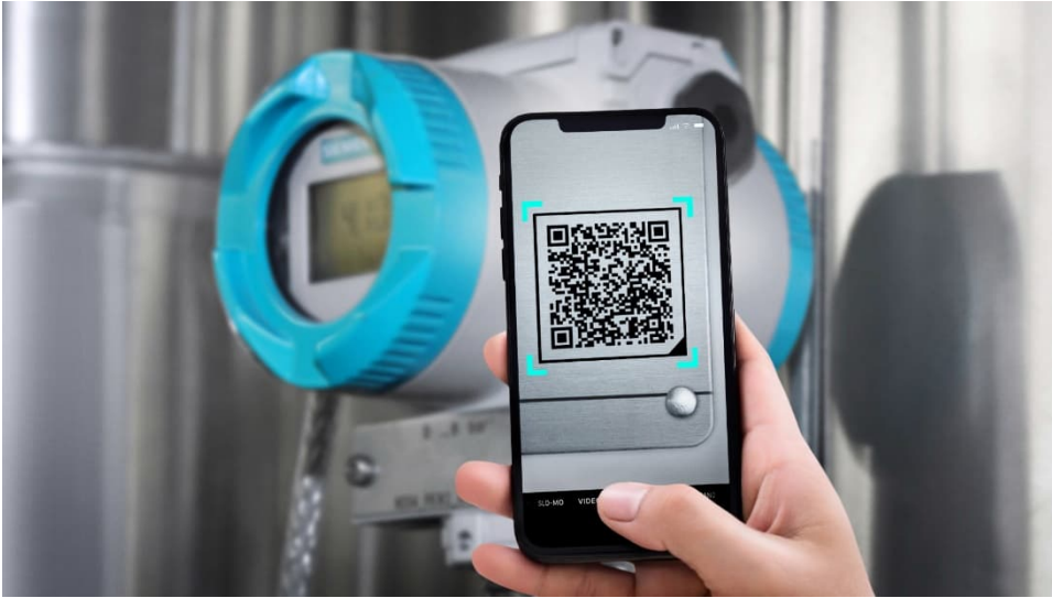
ID link on plant component can be scanned via mobile device
