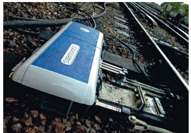
6ft points machine system
