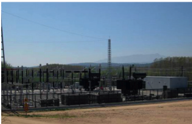
400kV/2x25kV traction substation
