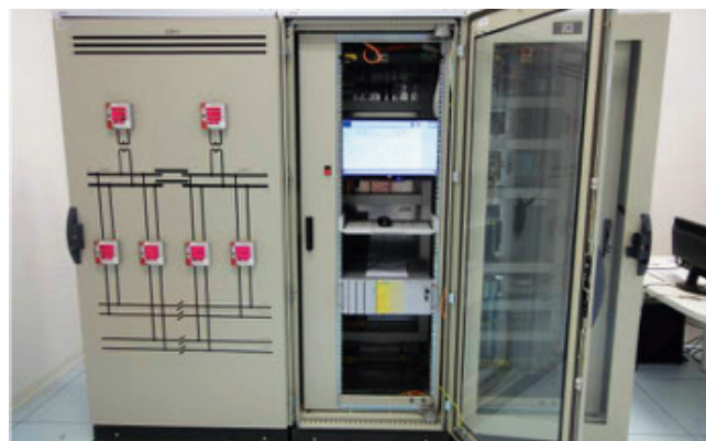
Local control panel at traction substation
