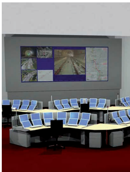
Picture of a tunnel control center with display wall
