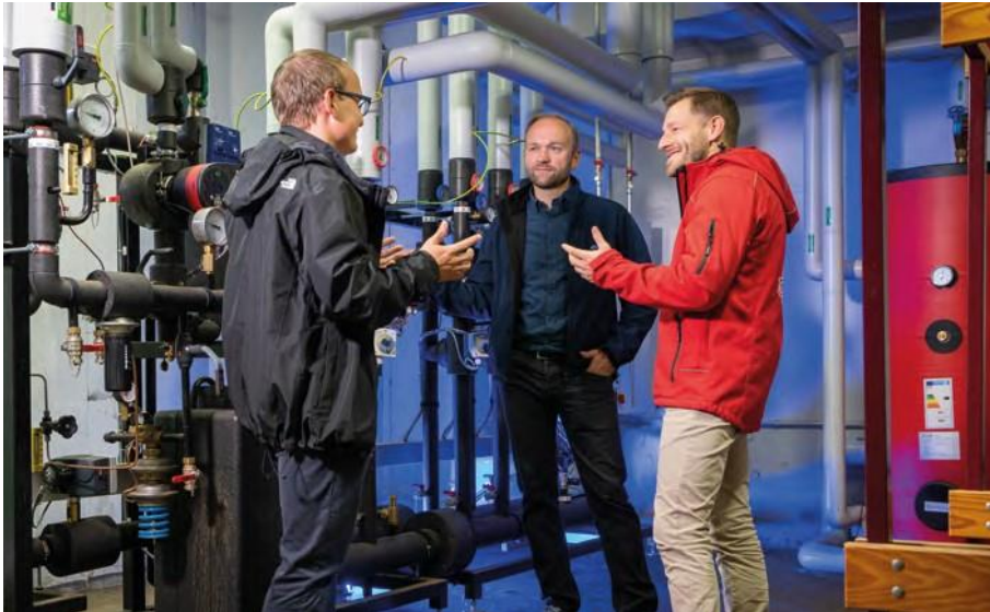
With the modern controller technology from Yados based on Climatix from Siemens, both the customer and the contractors are satisfied.
