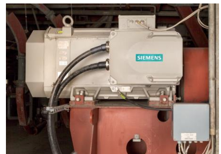
New speed-controlled SIMOTICS FD motor on the secondary fan
