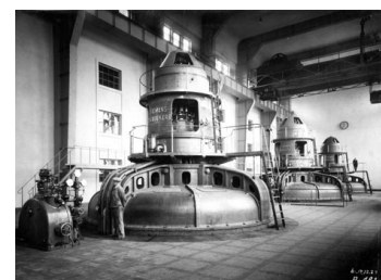
View of the generator hall, 1929
