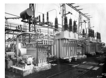
Outdoor transformer station, Inchicore near Dublin, 1930
