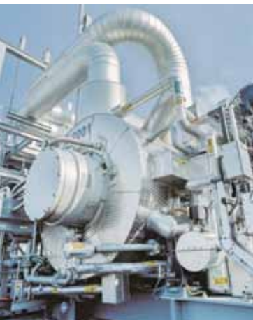
Air conditioning & compressors
