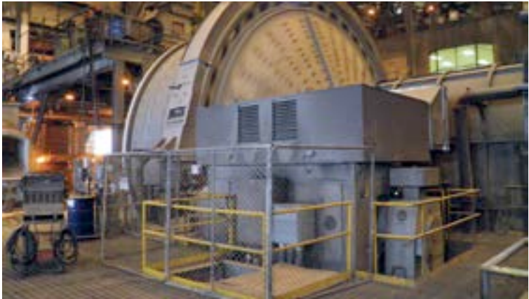
Conventional Mill Drives
