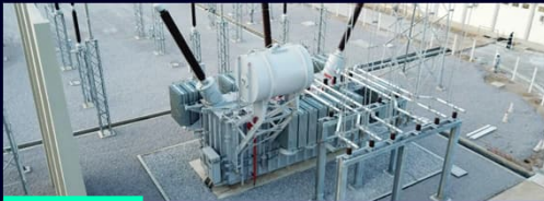
High Voltage Power transformers
