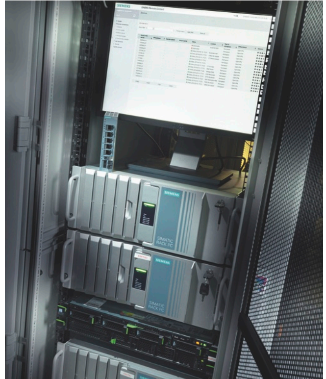
SINEMA Remote Connect and SIMATIC Rack PCs enable a secure and centrally managed VPN connection.
