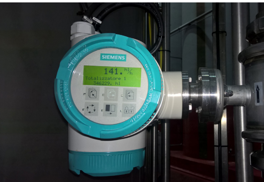
Siemens SITRANS F M MAG flowmeters and sensors monitor wine flowing from storage vessels to the bottling area.
