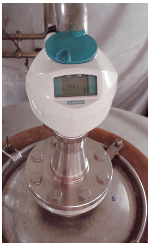
SITRANS LR250 radar transmitters continuously monitor levels of wine in Caviro's 124 storage vessels.
