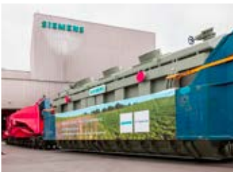
Large power transformers • Up to 300 MVA, 420 kV • Natural ester • Nuremberg 2013
