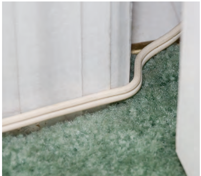
Damaged/bent cords can cause arcs
