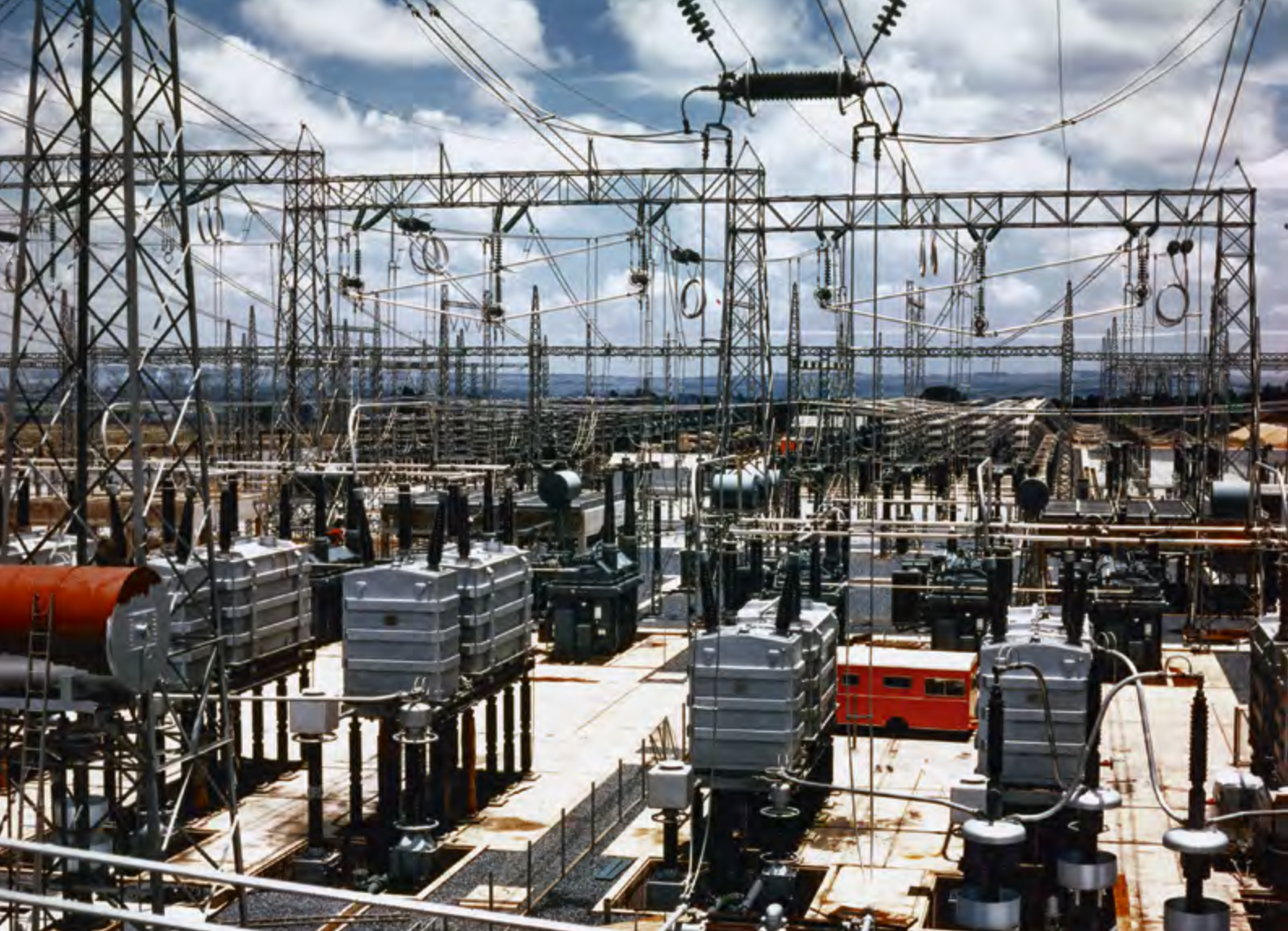
The HVDC transmission starting point: the Songo current conversion station near the Cahora Bassa power plant, 1975
