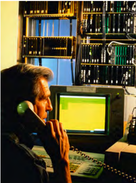
Deployment of the EWSD digital switching system at the telephone operating company Ohio Bell, 1988
