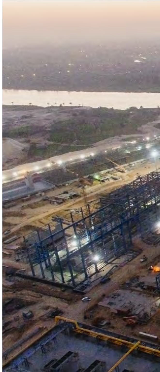
A combined-cycle power plant in Egypt, 2017
