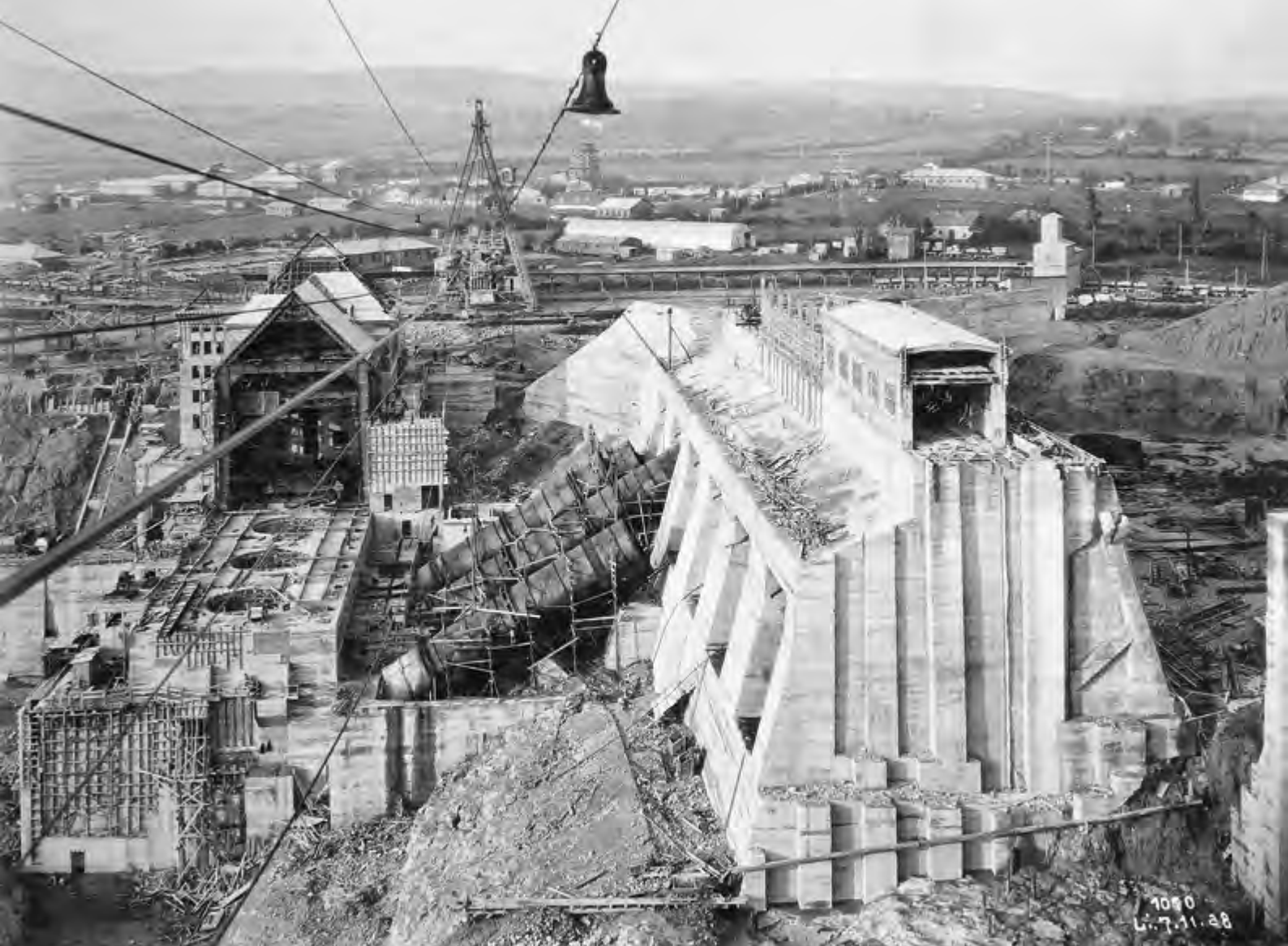
The Ardacrusha hydroelectric plant on the Shannon – building the generator hall and dam, 1928
