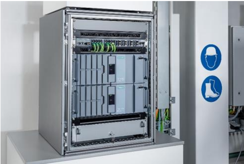
Private industrial 5G infrastructure for the deployment of a local 5G network
