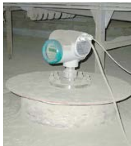
Fig. 3: Sitrans LR400 units such as this one were installed well over a decade ago, and continue to provide reliable level measurement readings to this day.
