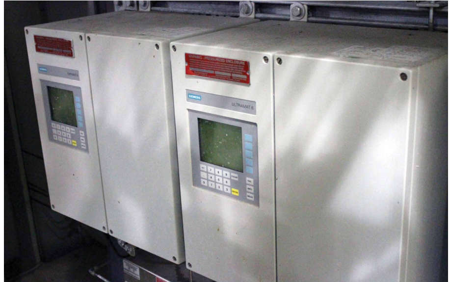
NCERC added a bank of OXYMAT and ULTRAMAT gas analyzers for measuring oxygen levels in the fermentation process.
