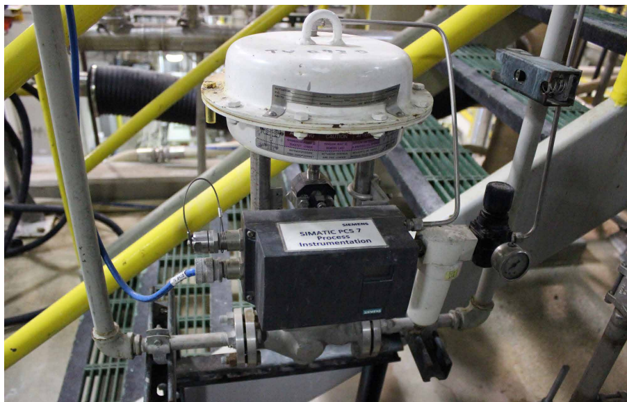
SIPART valve positioner on a carbon dioxide scrubber.
