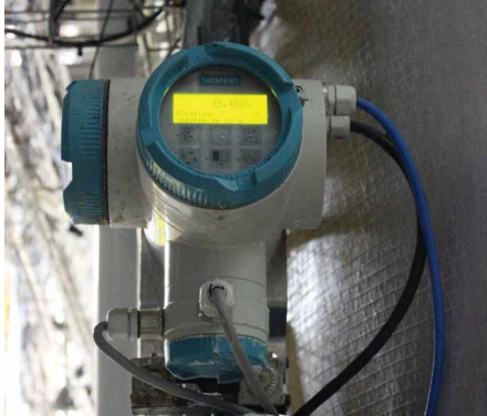
SITRANS FC Coriolis flow meter installed on a fermenter tank.
