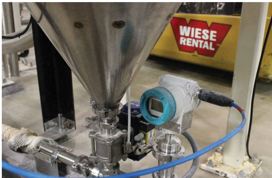
SITRANS P pressure transmitter monitoring the pressure in an eductor.
