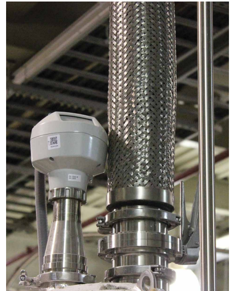
Level monitoring on the fermenters is carried out by SITRANS LR radar level indicators.
