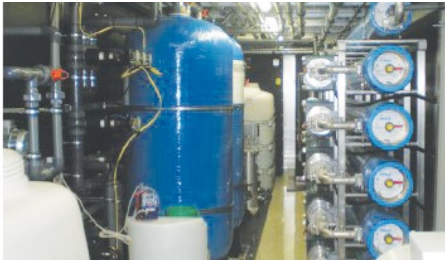
The membrane systems must be accommodated for in the narrow containers. The electrotechnical equipment must feature a "slim" design.
