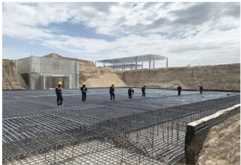
The accompanying images show construction work underway at Zarafshan, about 670km west of the capital city of Tashkent, Uzbekistan. All images courtesy of HORN Glass.
