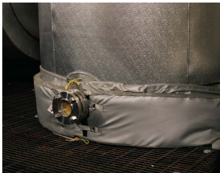
Kawartha Ethanol uses extra wraps of removable, customized insulation to reduce heat loss in crucial areas.
