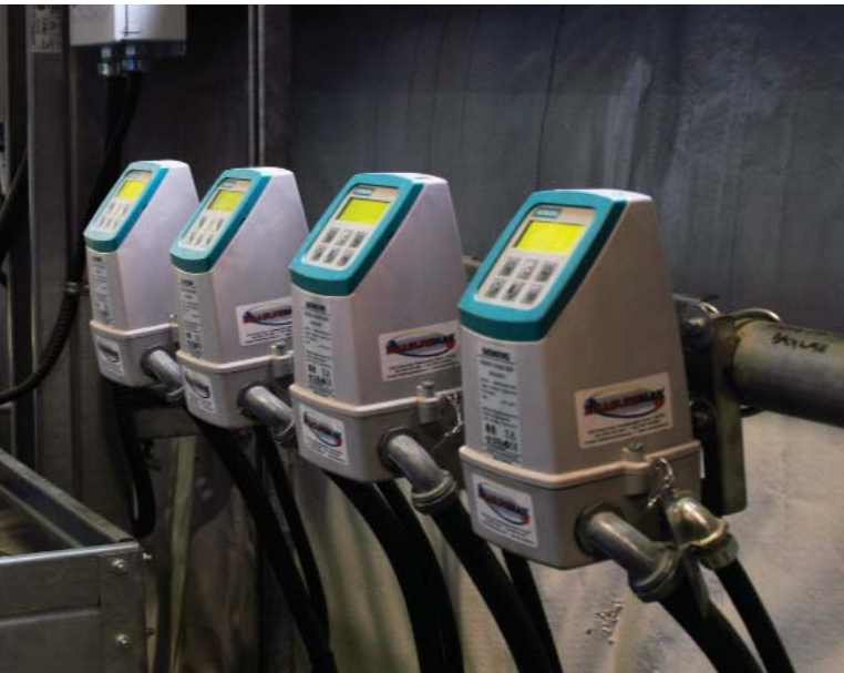
Dozens of Siemens flowmeters measure water, chemical dosing, and material flow throughout the ethanol production.
