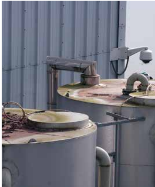
Two SITRANS LR250 radar transmitters monitor the levels of storage wastewater feeding the digesters.
