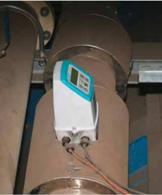
SITRANS F M MAG 3100 flowmeter monitors the Percolate flows.
