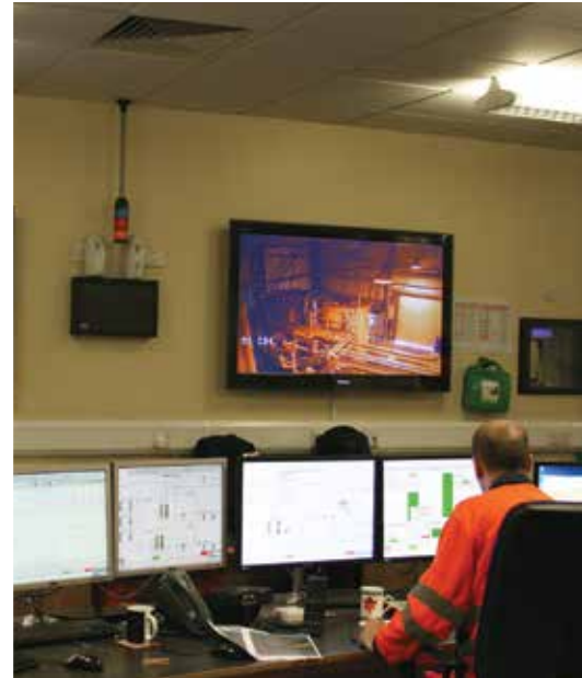
Using a SIMATIC WinCC SCADA System, operators monitor and control the entire facility from a central control room.
