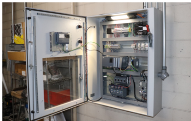
The SIMATIC S7-1500 PLC, SIRIUS soft starters, and other system components are located in a nearby utility room.
