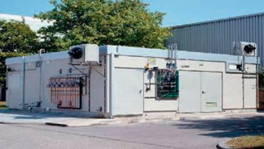
Fig. 11: Analyzer house (shelter)
