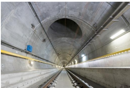
Image 3: Fire detection by Siemens: thermal imaging cameras, smoke detectors, and Fibrolaser
