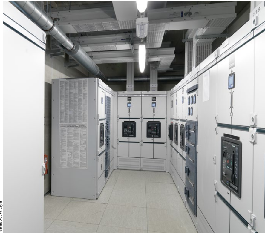
The low voltage is transmitted to the loads through Sivacon S8 switchgear and Sivacon 8PS busbar trunking systems
