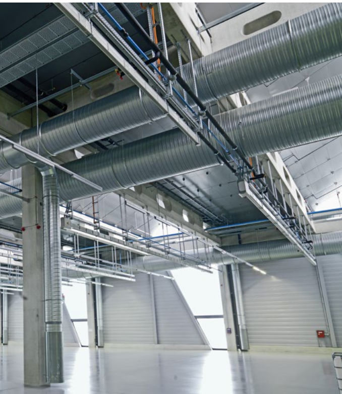
The new production halls of Hawe Hydraulik feature state-of-the-art building management systems
