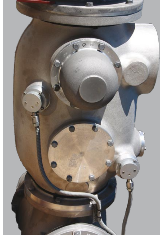
Fixed mounted cameras on the disconnecter and earthing switch module
