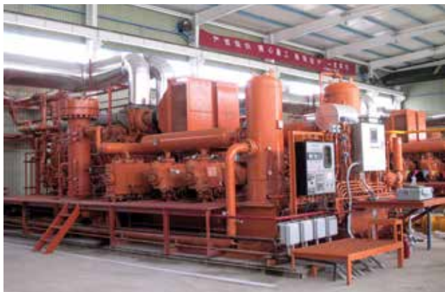
Six-throw HOS compressor installed in China.
