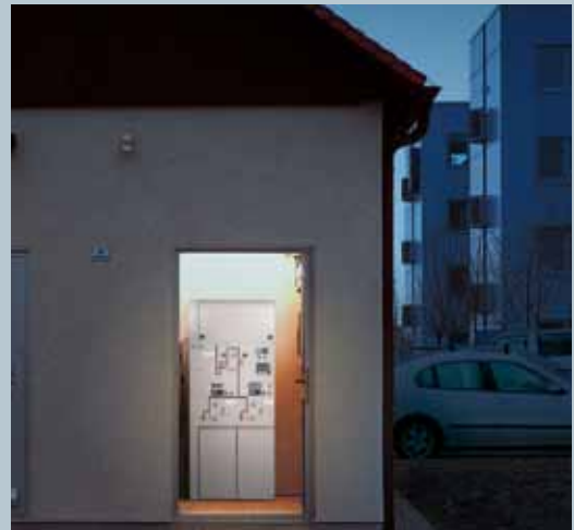
Retrofit – optimum design for effective utilization of switchgear rooms
